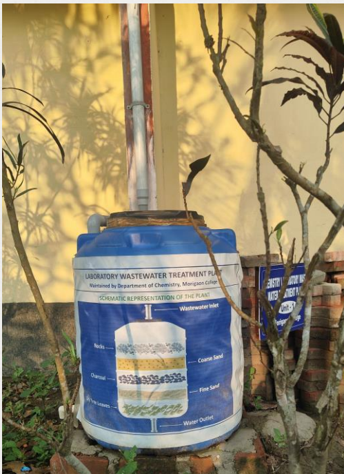
Laboratory Waste Water Treatment Plant
